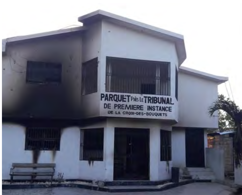
Fire damage to the Croix-des-Bouquets court of first instance building after a criminal group set it on fire in July 2022. © 2022 Private.
